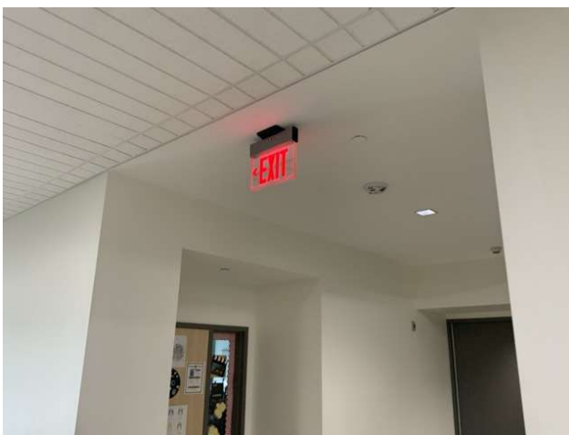
35 - FIRE ALARM SYTME DEVICES
