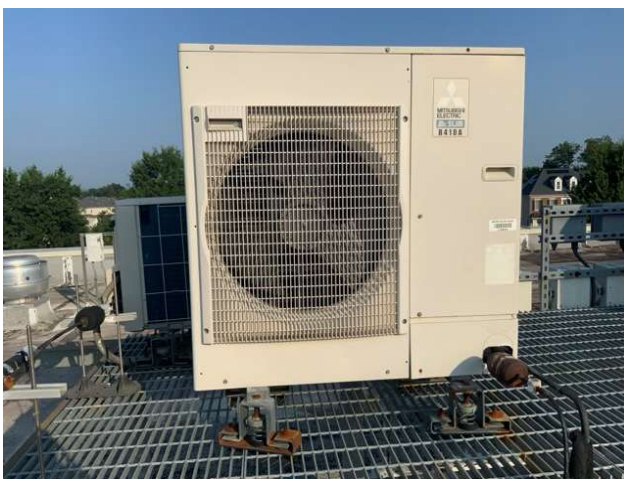
23 - SPLIT SYSTEM DUCTLESS
