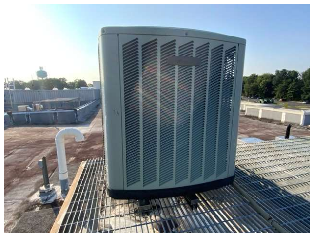
24 - SPLIT SYSTEM (CONDENSER)
